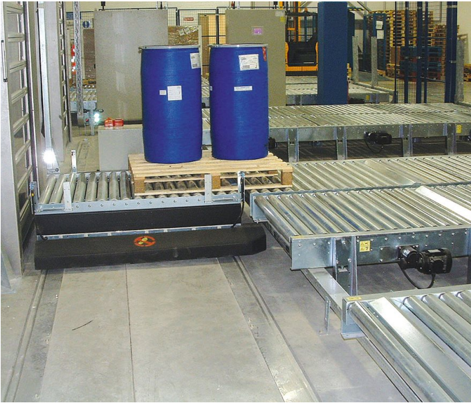
Transfer trolley installed in a pallet roller conveyor system supplied to Organon, Ireland.
